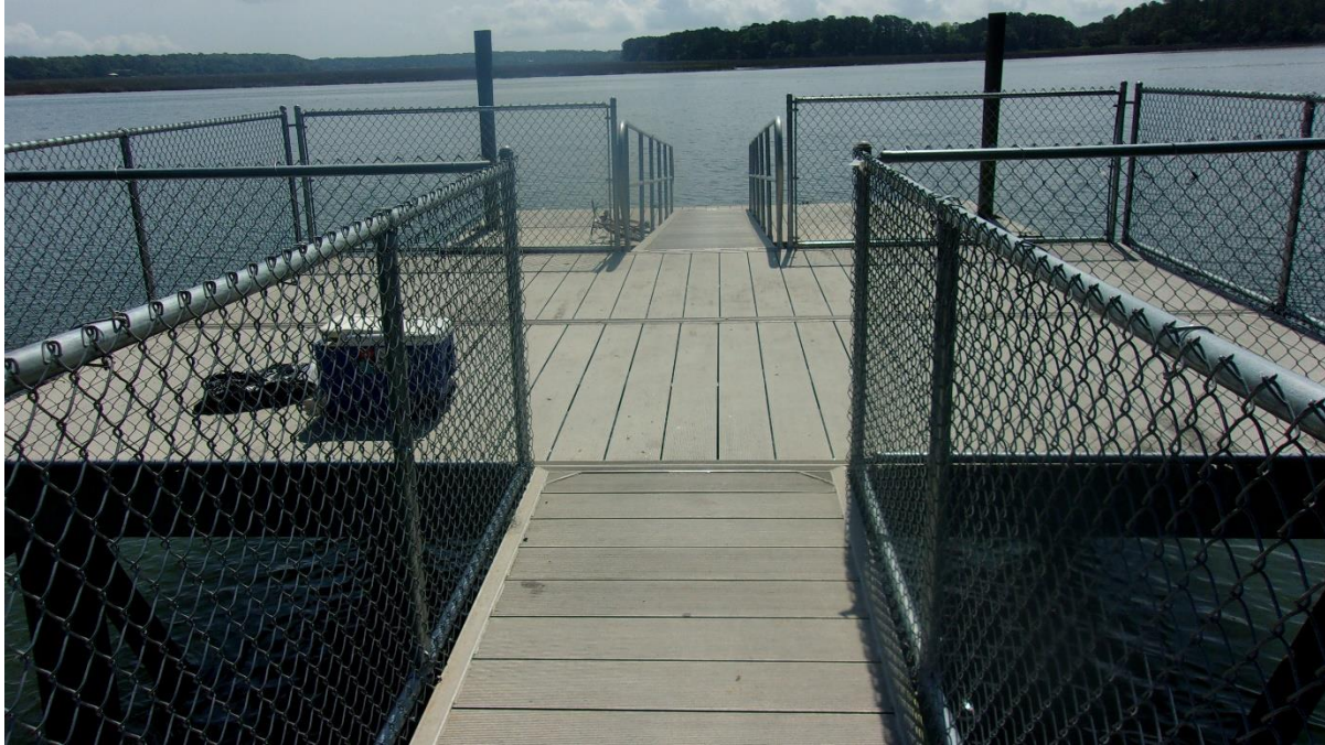
Dock, observed to be in good condition Note metal surfacing, aluminum railings
